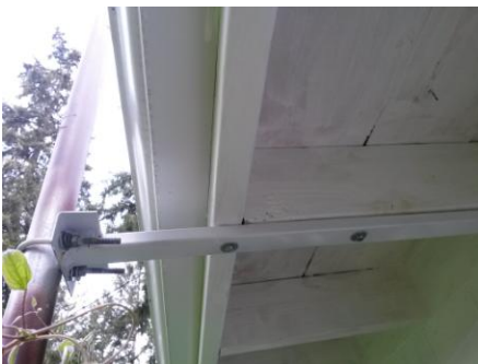
Mounting to house and avoiding gutter
