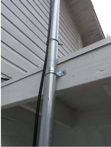
Mounting to house of 40' pole. Fastens to house in two locations, one at the lower roof (shown here) and a second on the second story roof..
