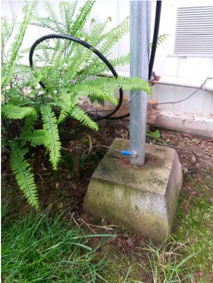
Base for permanent mounting, note service loop in conduit and ground wire to 8' copper clad ground rod
