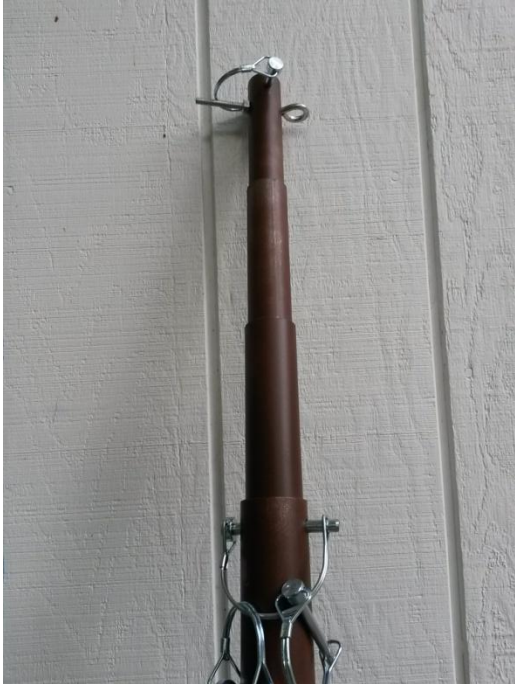
Top of collapsed pole
